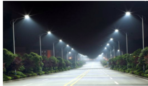
50,000 street lights and 6000 sign lights
